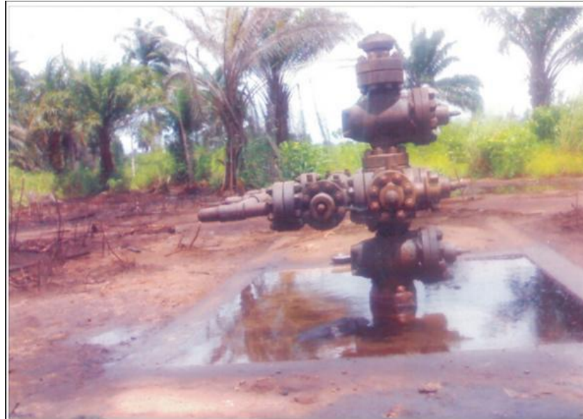
Figure 1: Ibibio 1 corkscrew well at Ikot Ada Udo
