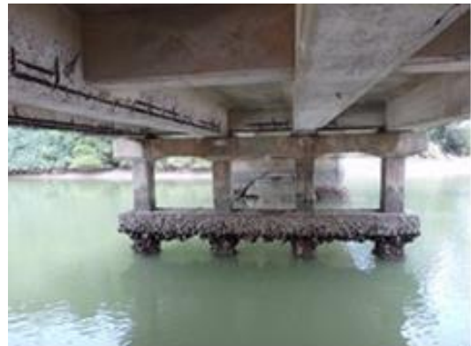
Fig.1. RC Bridge deteriorated by salt attacked
