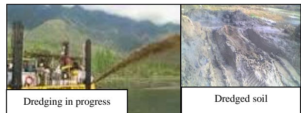
Fig. 1. Dredging of Dal Lake in progress and accumulation of dredged Soil along Lake Shores
