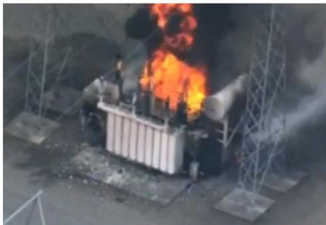
Fig. 2. Example of transformer failure with fire
