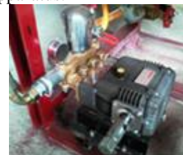
Figure 3. Water pump and main valves
