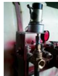
Figure 1. First electric valve
