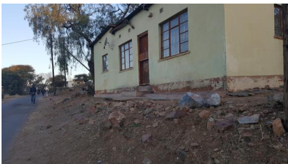
Fig.8. Image showing inadequate setbacks between front building and road frontage
