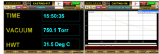
Fig 10 – Casting SCADA Screens
