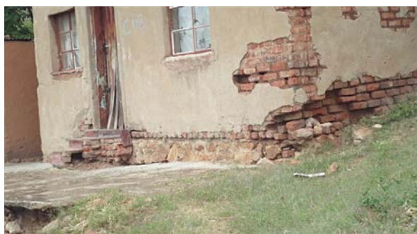
Fig.13. Image showing cracks on building as a resultant of developments not regulated by Engineers
