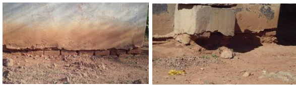
Fig.9. Images showing buildings damaged by floods
